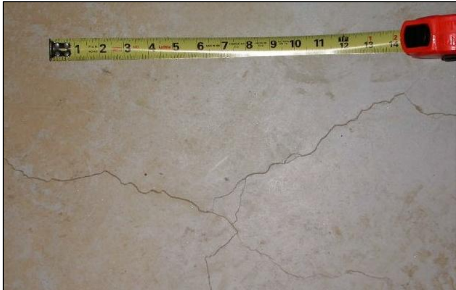
Figure1.9 Minor cracks on floors of ground floor
